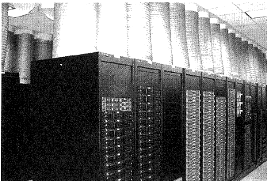
Figure 6: High-density containment systems installed in data center.
